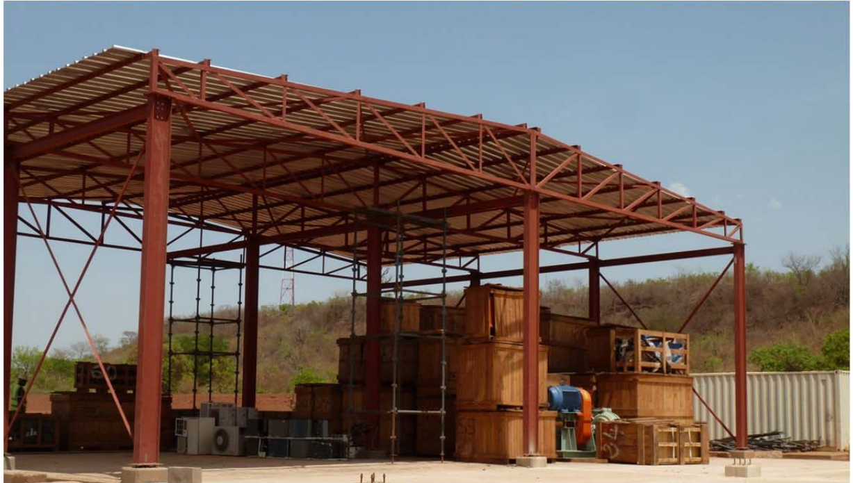
Power House for Generators
